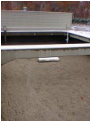
The objective of the decanter is to remove the supernatant from the SBR minimizing the discharge of suspended solids or foam.
