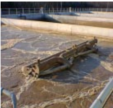
At this plant in Ontario, there were no connecting pipes between the SBRs. For this reason, the MLSS had to be transferred from a tank to be serviced to one in operation using portable transfer pumps. Notice lack of access (walkways) to tanks located in the centre.
