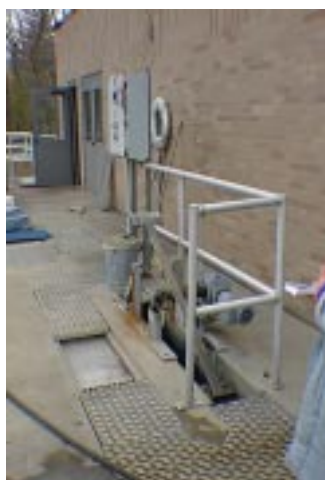
This underdesigned screening system at this 1700 m 3 /d SBR plant caused wastewater overflows under high flow conditions.
