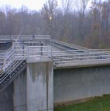
At this plant in Ohio, this uncovered and elevated reactor had lower water temperatures than the contiguous and less exposed reactors.
