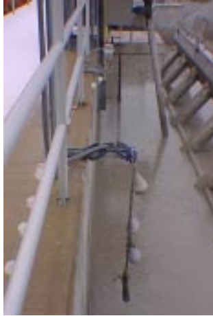
At this plant in Michigan, floats were preferred over other level sensors for their simplicity.
