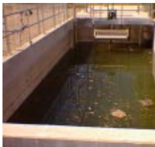
Pre-treatment equipment with poor performance caused accumulation of floatables at this SBR facility in Ontario.
